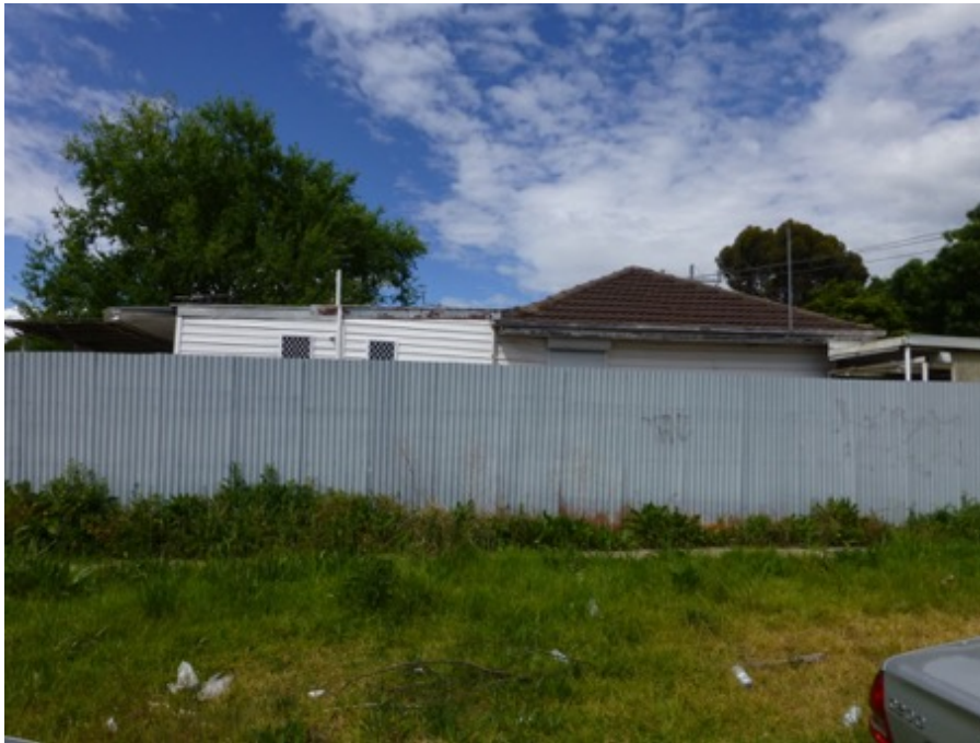
Figure 28 Group 3 Half-house attached to the rear of a weatherboard and tile house. Source, heritage Alliance 2019
