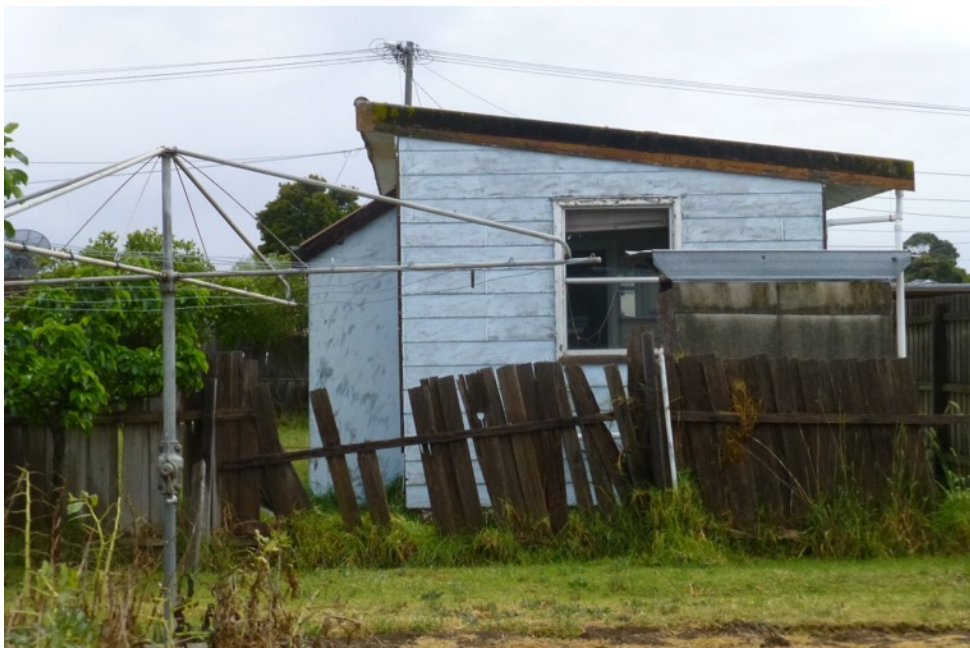
Figure 22 Southern Façade from backyard with outside toilet in asbestos cement sheet and intervening split paling fence. Source, heritage Alliance.
